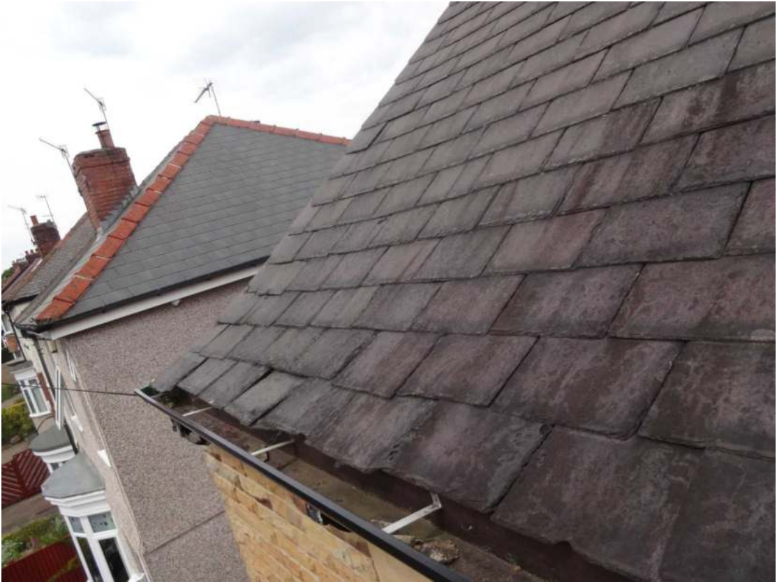
loose slates to roof
