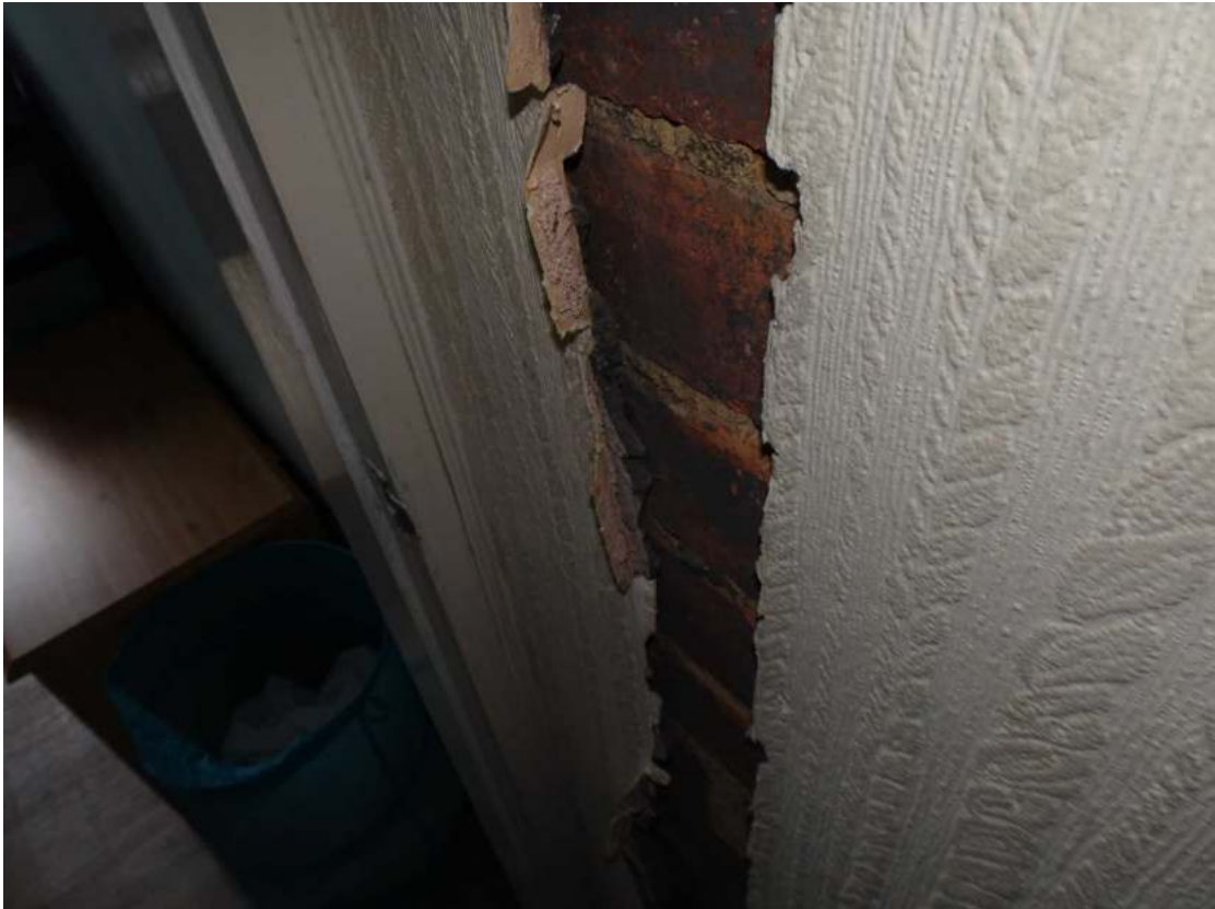
Some areas of loose plaster
