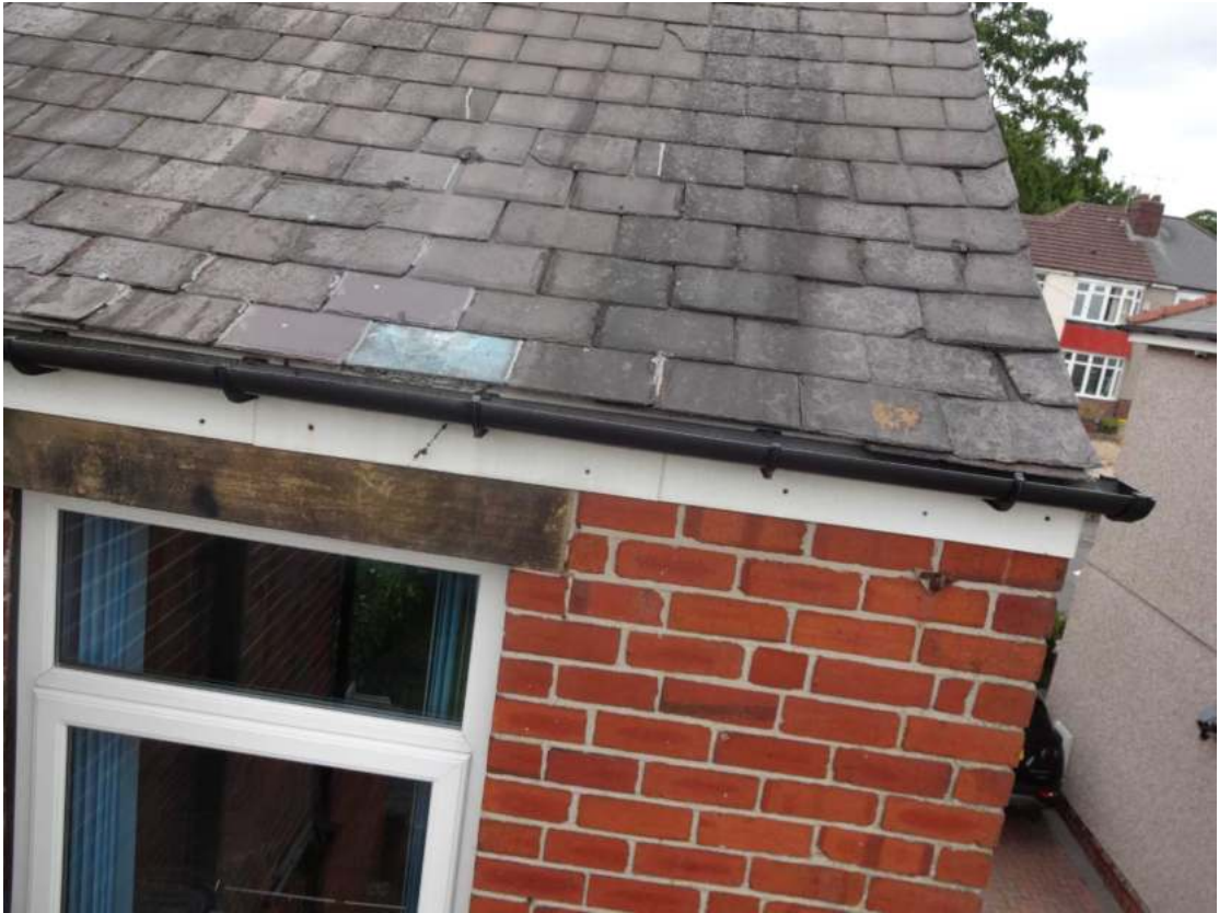
loose and damaged slates
