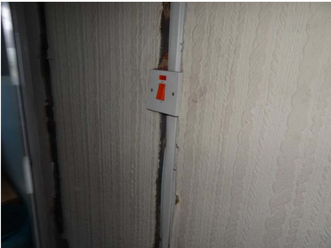
Plaster repairs required
