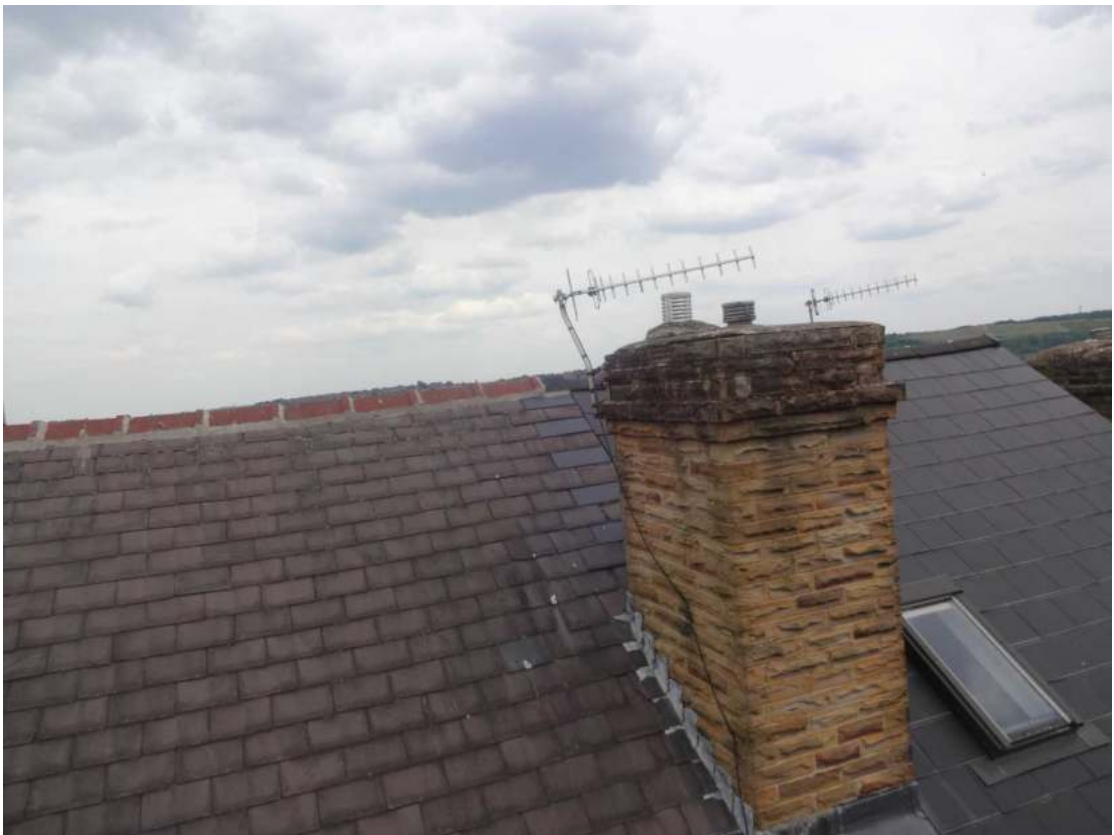
Cracked flaunching' around terminals and pointing
