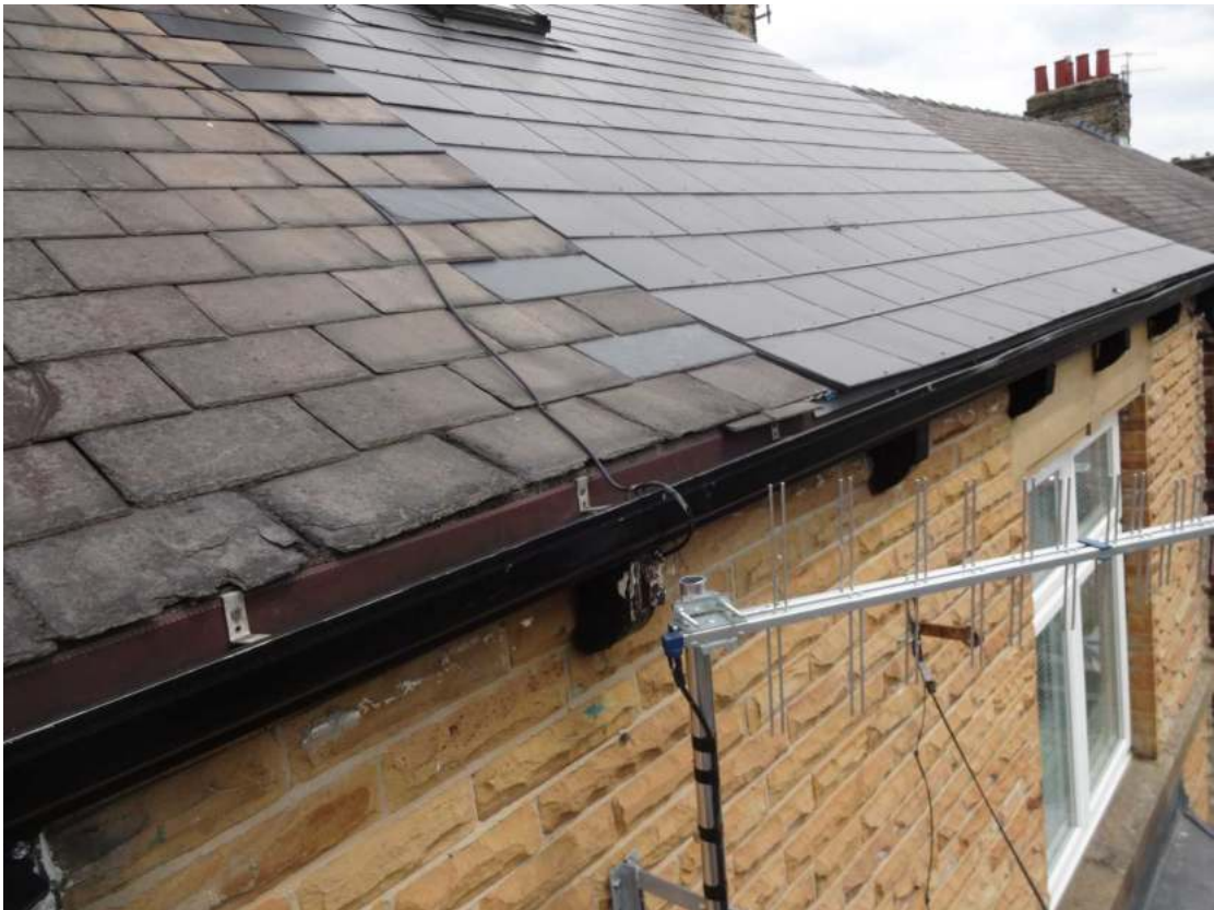
Slates short of gutter, fix eaves tray
