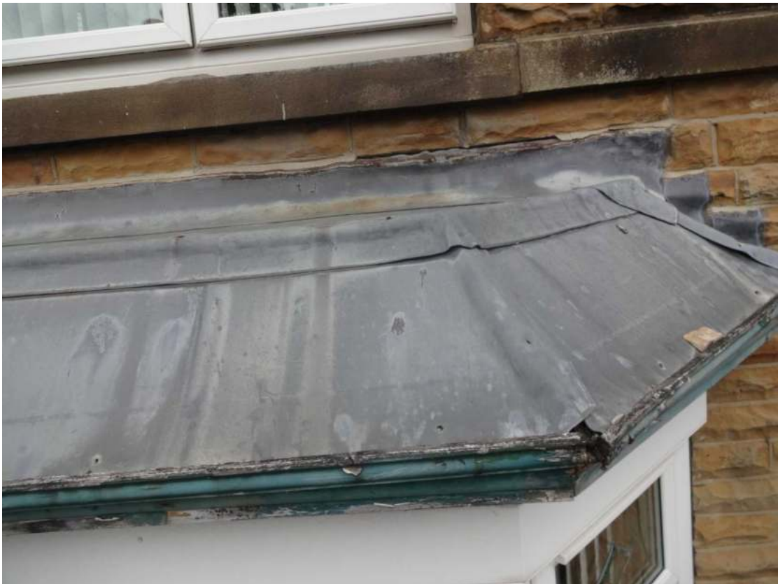
lead flashing loose to bay top
