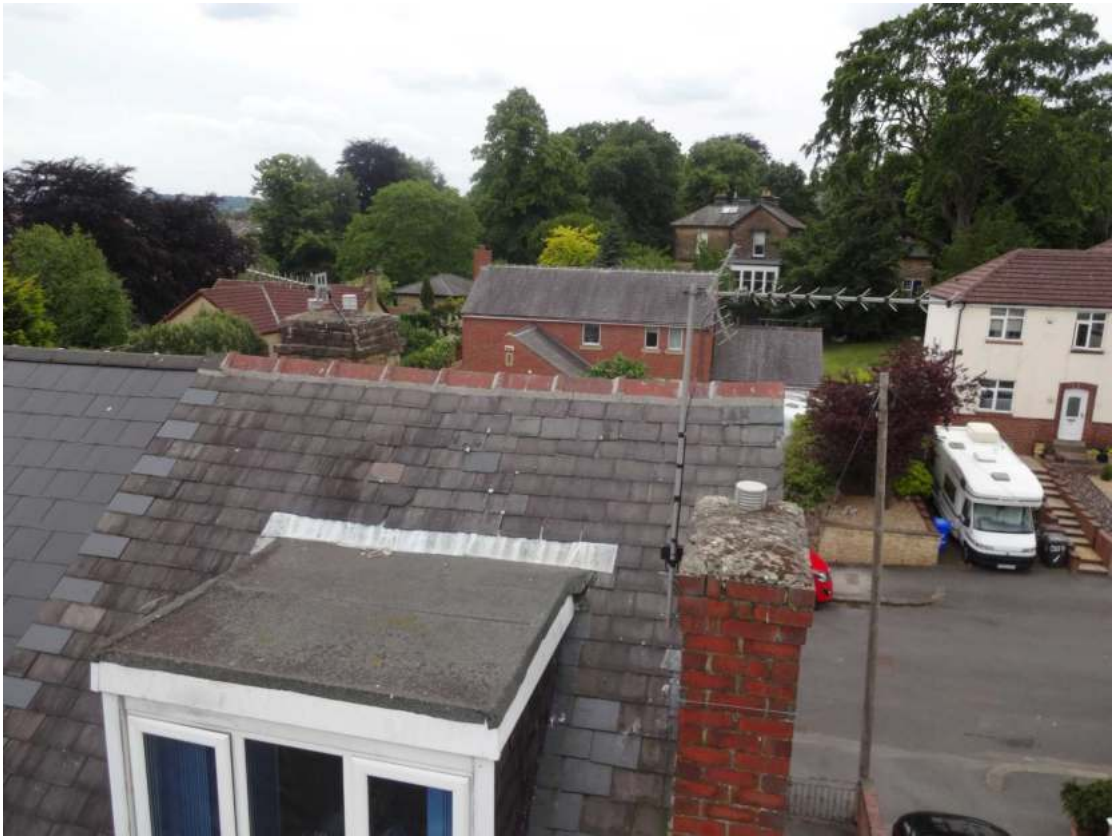
Cracked flaunching around chimney terminals
