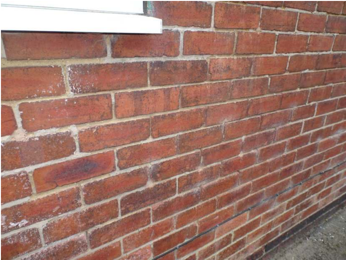
Areas of repointed needed in future
