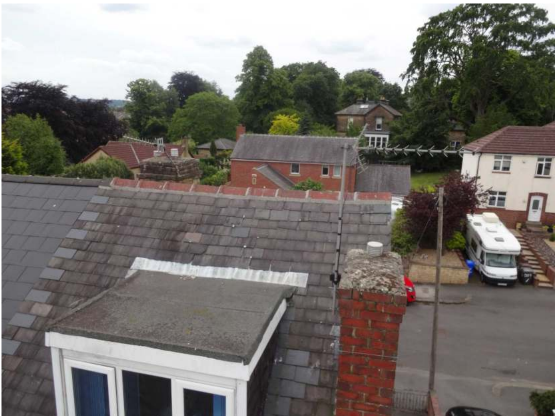
Dormer top covering is untidy and poorly fitted
